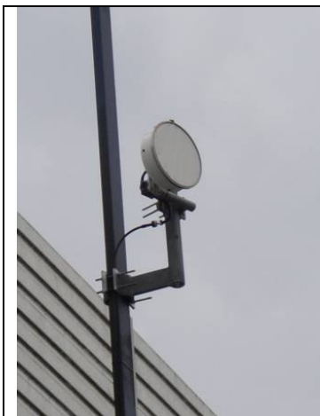
Figure A4.7: FS antenna B at bridge
