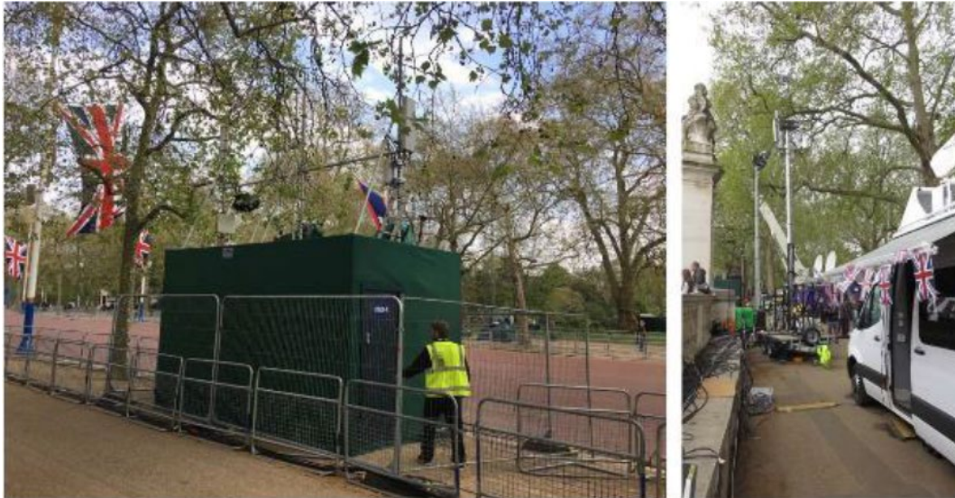
Figure 16: Antenna arrangements for Cell 2 (“The Mall”) and Cell 1 (“Green Park”)
