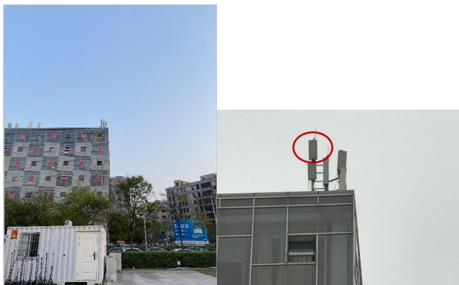
Figure 8: 5G NR base station
