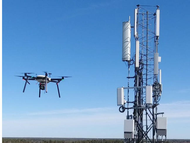
Figure 11: 5G NR base station
