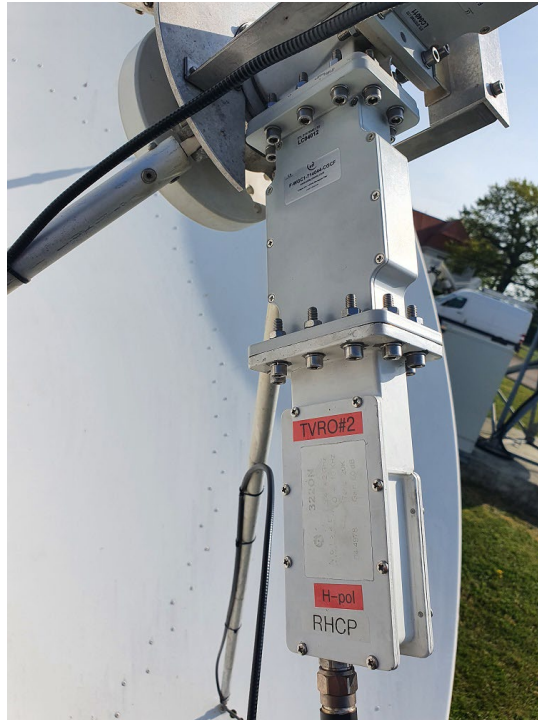
Figure 5: Sample of an FSS earth station with the ETL filter installed
