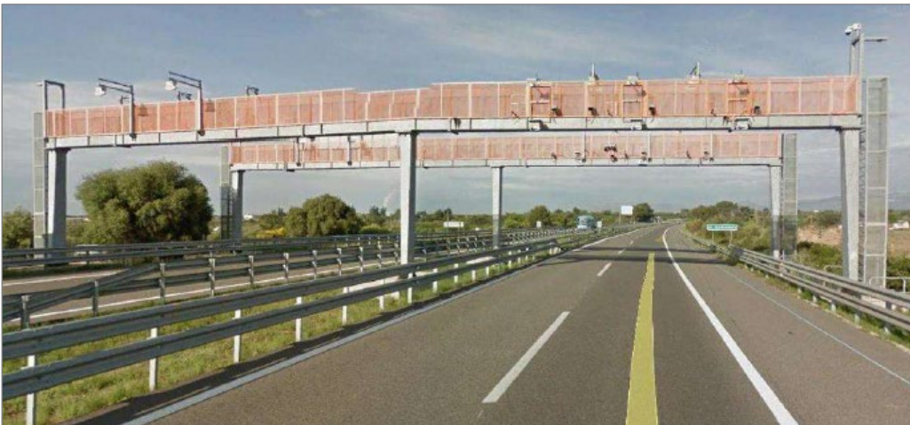
Figure 4: Free flow toll gantry on the Spanish motorway AP-7
