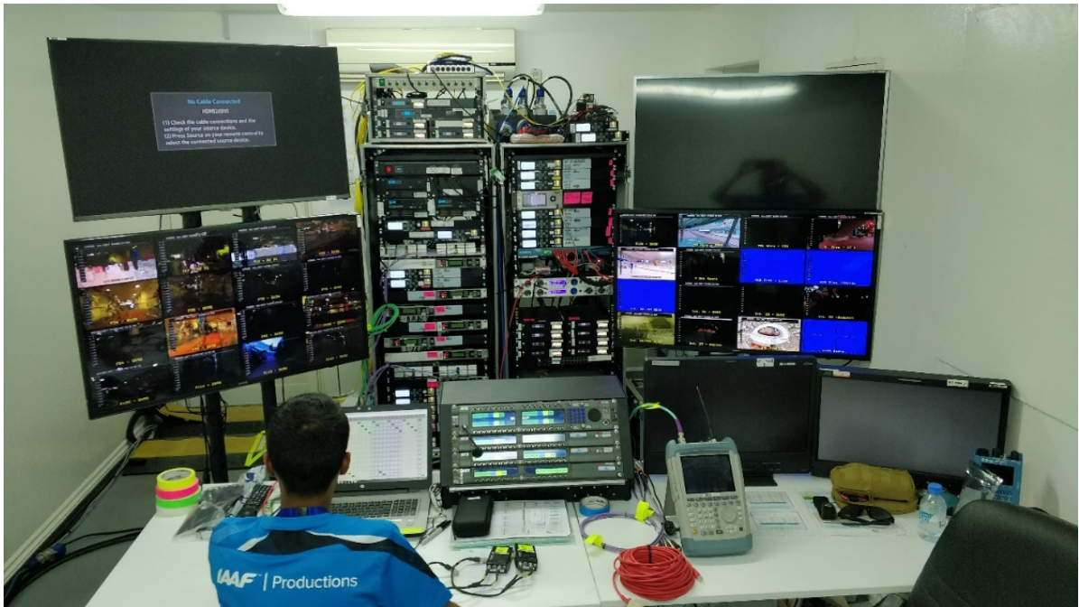
Figure 15: Temporary control room
