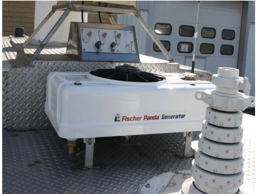
b) Diesel engine cooling radiator, located on the vehicle roof
