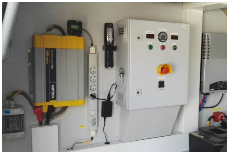
Figure 28: Power supply system control unit (Serbia)
