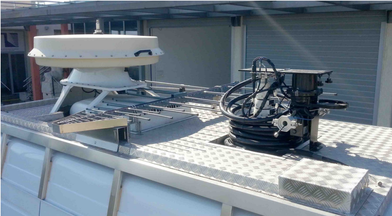
Figure 17: Coiled antenna feeder and rotator supply cable (Montenegro)
