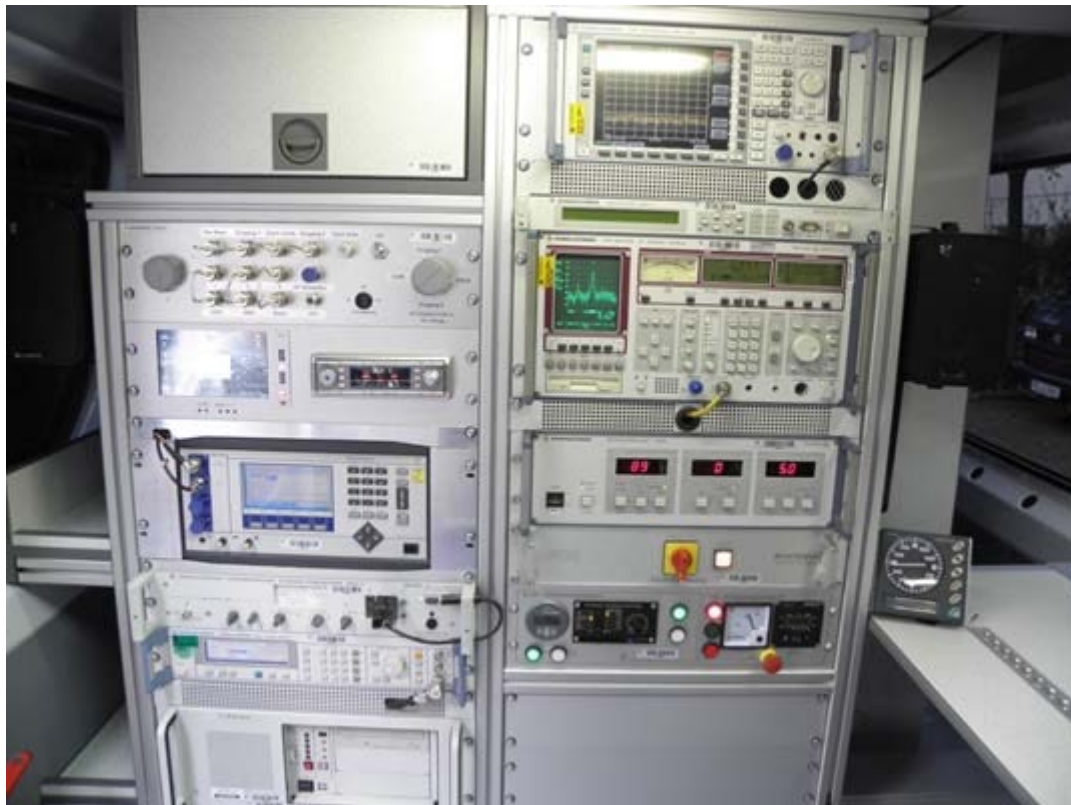
Figure 23: Arrangement of measuring, monitoring and additional devices in standard racks (Germany)
