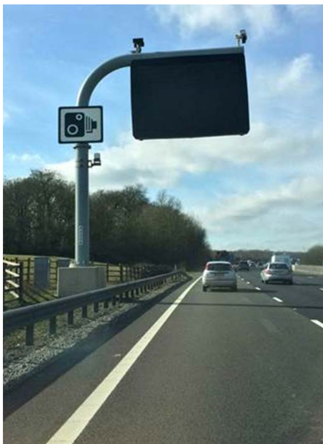
Figure 13: Example Fixed Radar Installation Location
