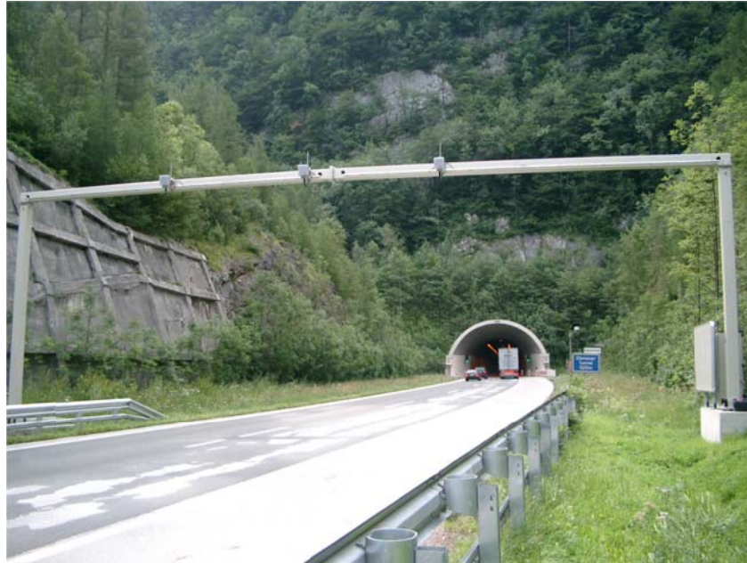
Figure 10: Typical free-flow installation with three lanes
