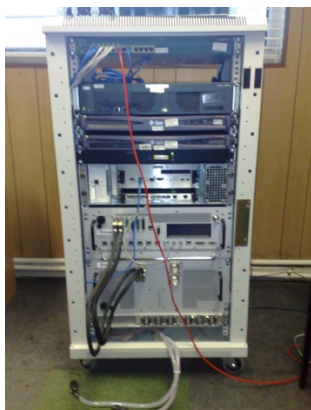
Figure 27: Ground Station Equipment
