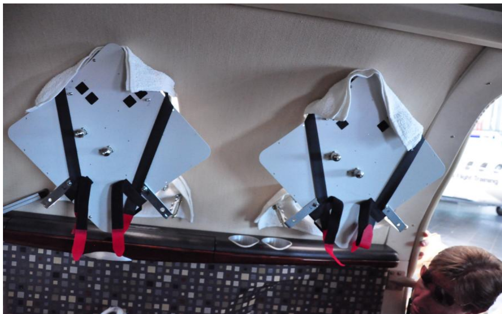
Figure 23: DA2GC Aircraft Station antenna mounting arrangement
