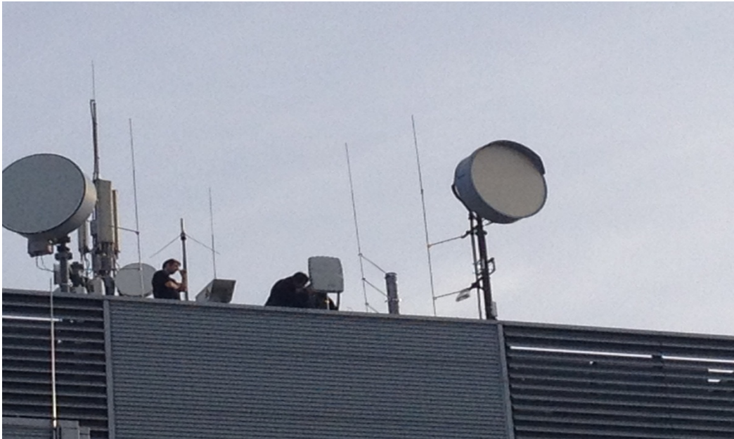
Figure 22: DA2GC Ground Station mounted on roof top
